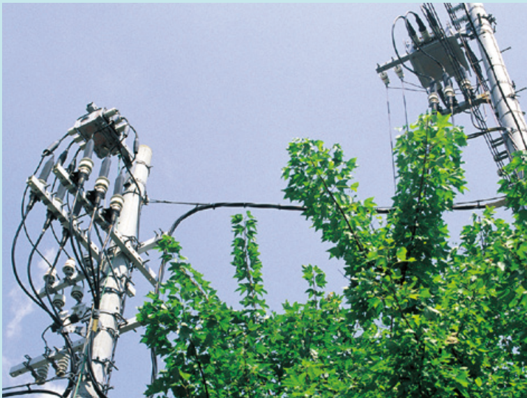
▲ 6kV終端接続材 6kV terminations as installed
