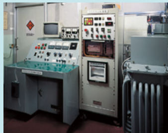
▲ AC耐電圧・コロナ試験室 Laboratory for tests of AC insulation strength and corona
